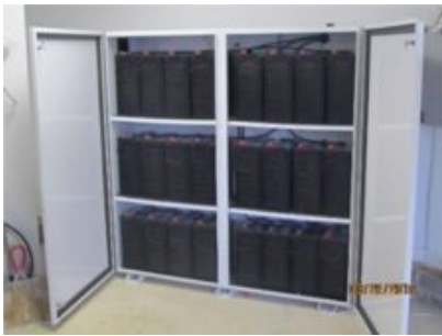
Batteries and Enclosure
